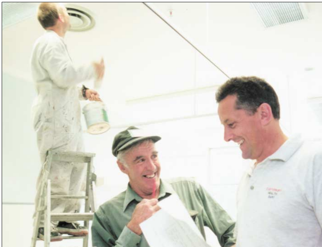
The builders' foreman, Barry Allport, and Christchurch Hospital building maintenance supervisor, Gary Busch, discuss the renovations programme.
